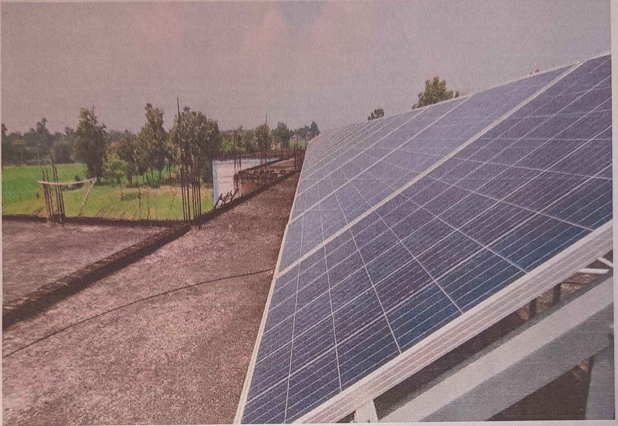
Solar plate installed in the roof top of main building
